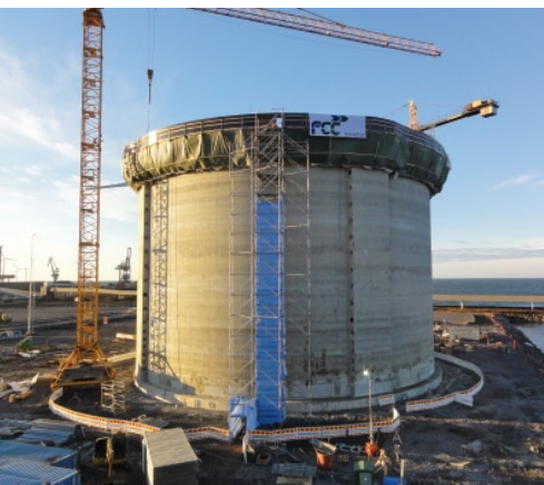
Tanque GNL, Finlandia
